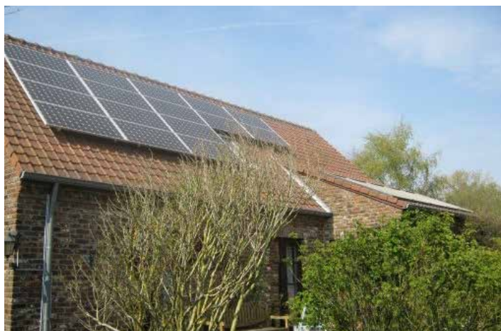
Installation photovoltaïque 4 kW
